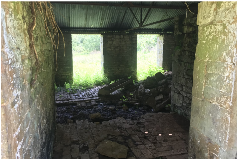
Internal view of derelict barn.
