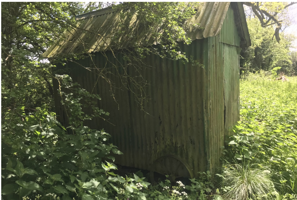
View of corrugated metal shed on northeast boundary of Area 1.—northern area of site.
