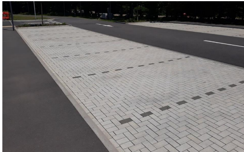
Figure 14: Example Image of Permeable Concrete Block Parking Bays
