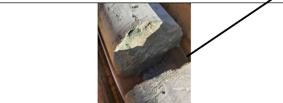
Photograph 2c: Green staining on the limestone
