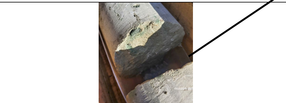
Photograph 8c: Green staining on the limestone
