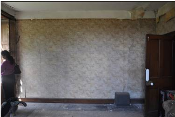
Photograph shows the wall where the opening is proposed. We have not checked the skirting to the principal room for evidence of piecing in.
