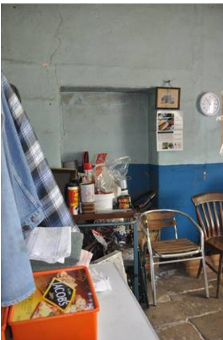
Photograph shows a possible blocked opening but it may have just been a shallow cupboard or niche for shelving – there is ghyssing for bracketed shelves. This is not shown on the survey plan.
