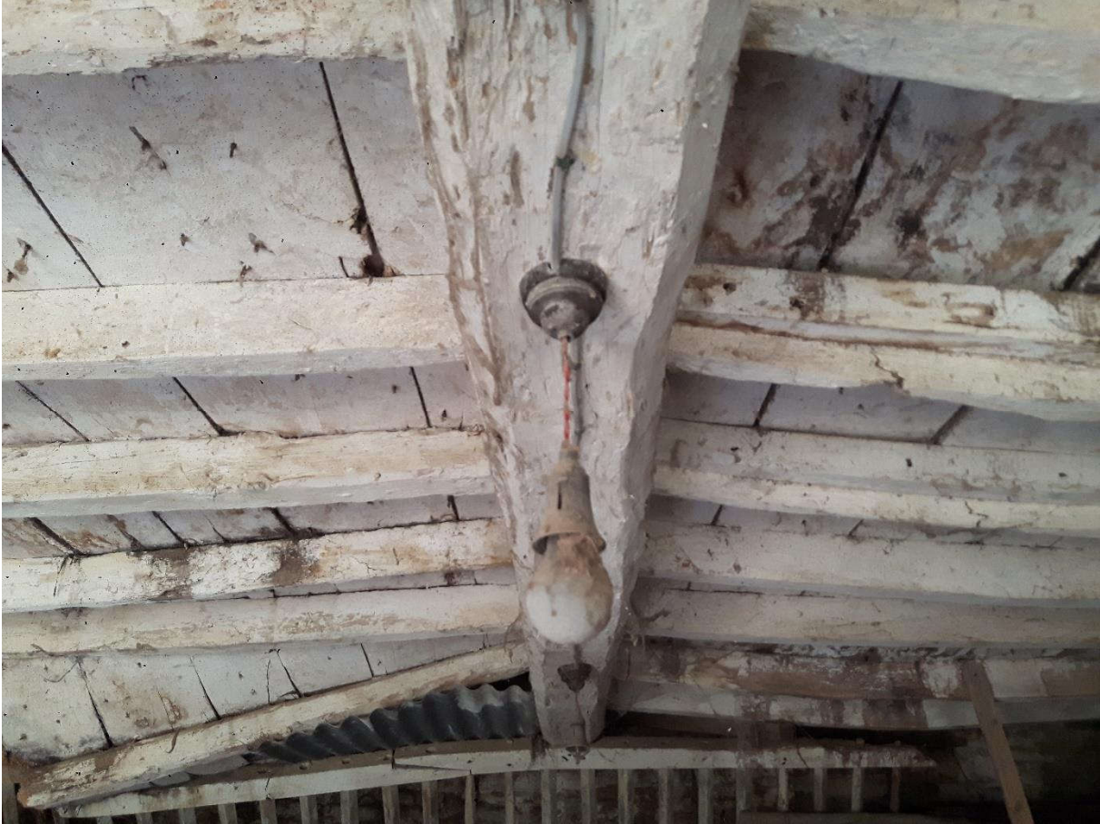
Photograph 24 - Block B, bridging beams and collapsed floor joists
