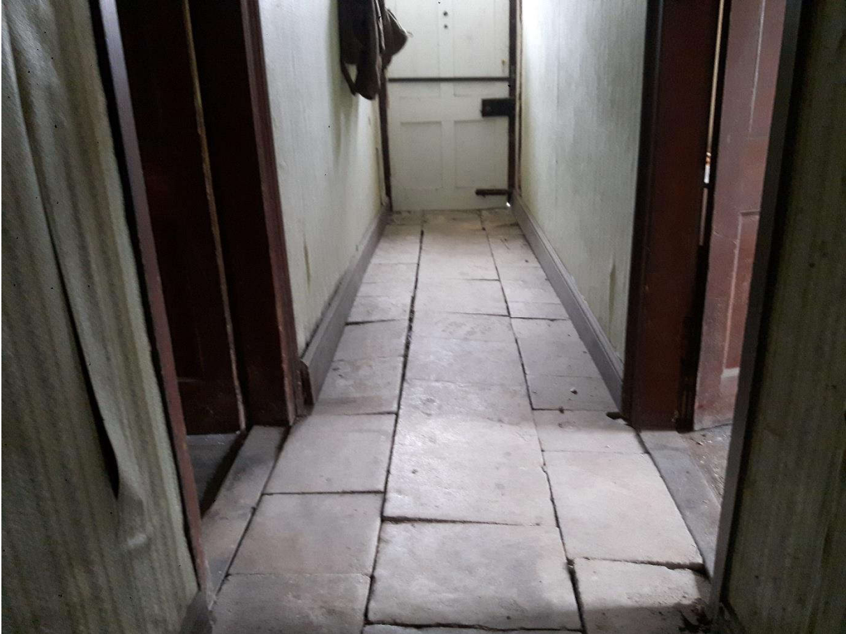
Photograph 9 - Main hallway fall towards west
