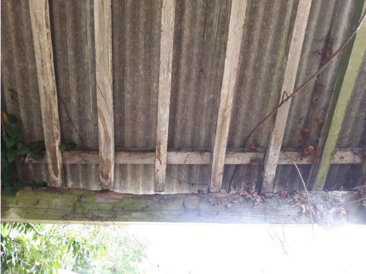
Photograph 35 - Block F, dropped eaves beam separating from rafters
