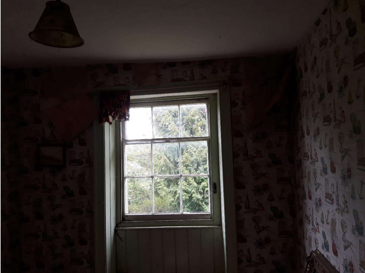
Photograph 13 - Internal lintel in south wall, central window over front door
