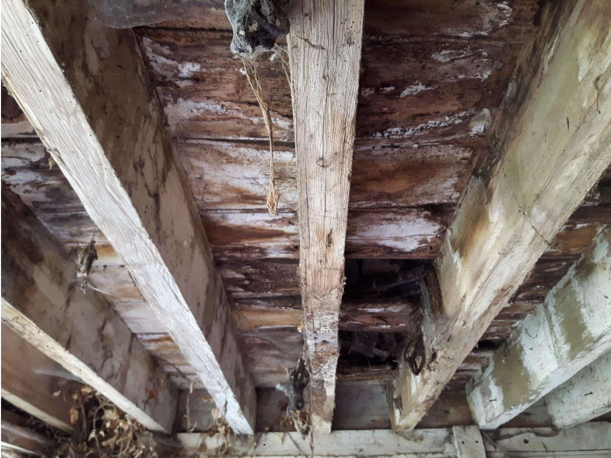
Photograph 20 - Block A, mezzanine timber joists, with rot damage
