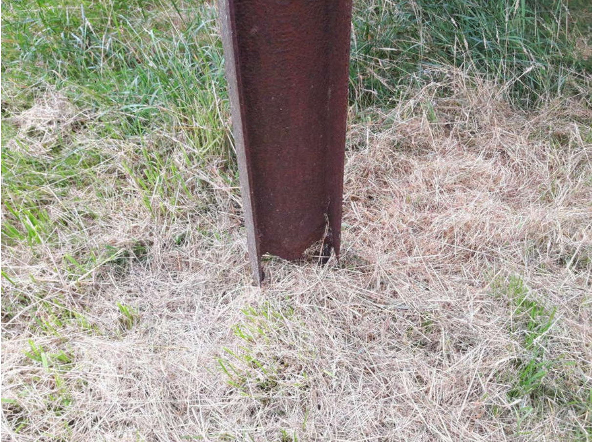
Photograph 29 - Block D, column base corrosion
