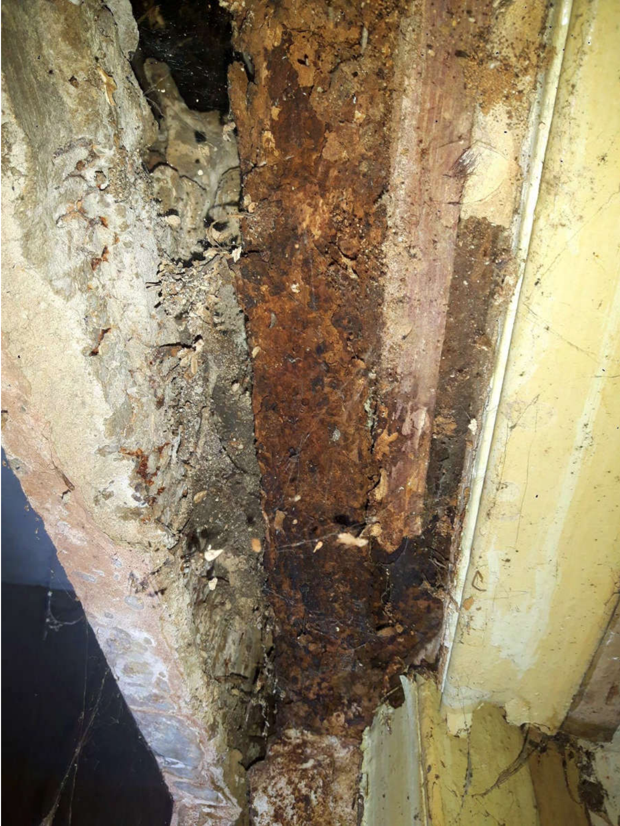
Photograph 14 - Rotten timber beneath gap between roofs
