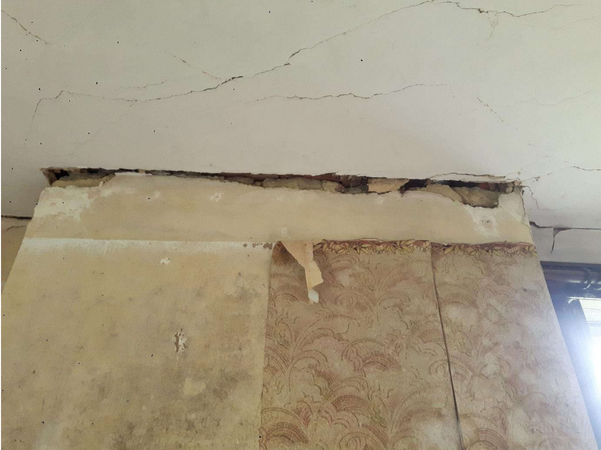
Photograph 10 - First floor joist separation from west wall from below
