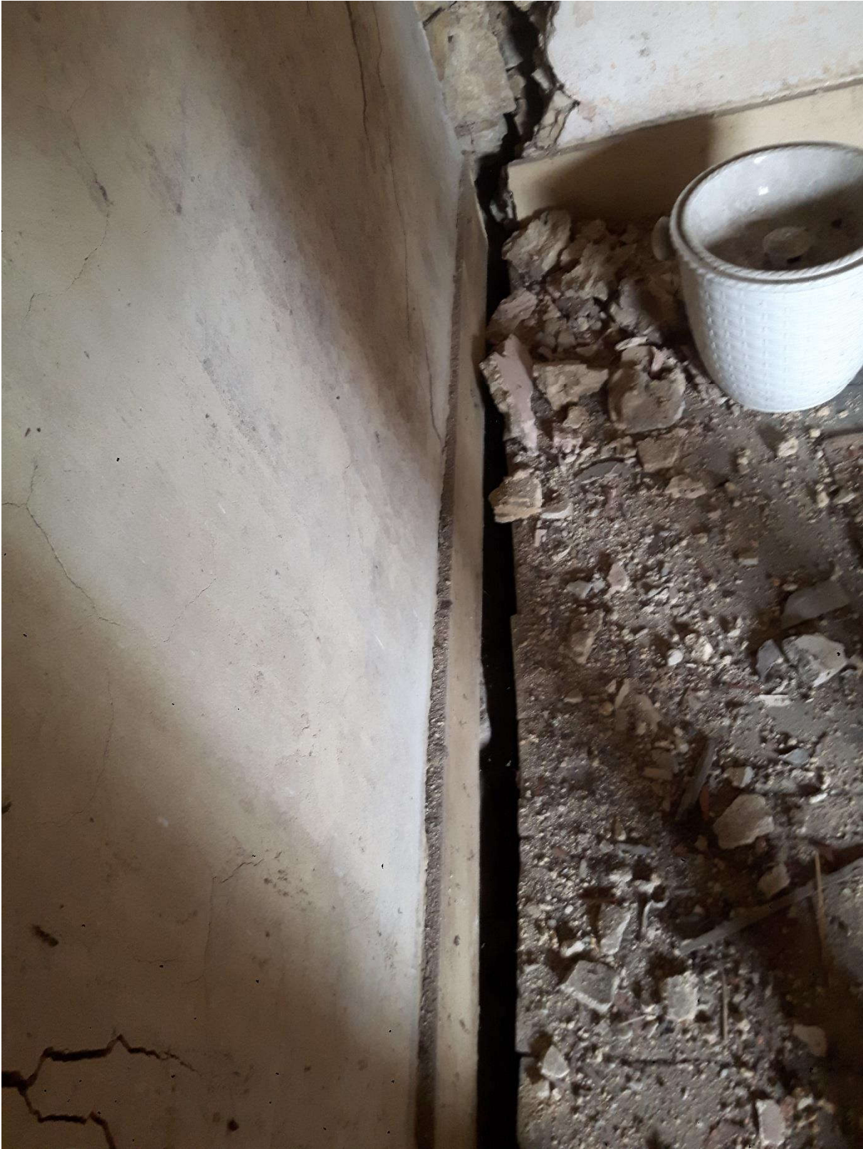
Photograph 11 - First floor joist separation from west wall from above
