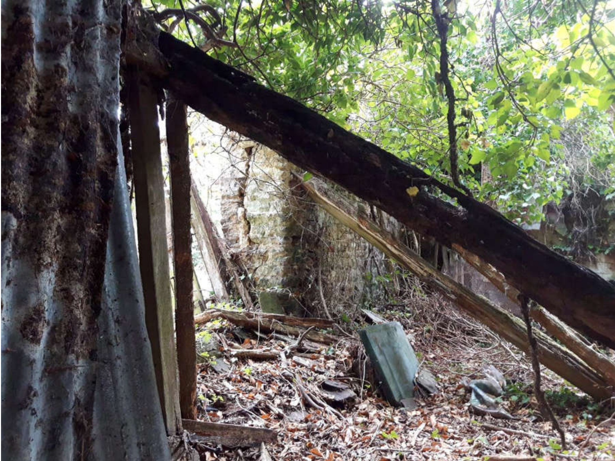
Photograph 36 - Block F, south roof collapsed
