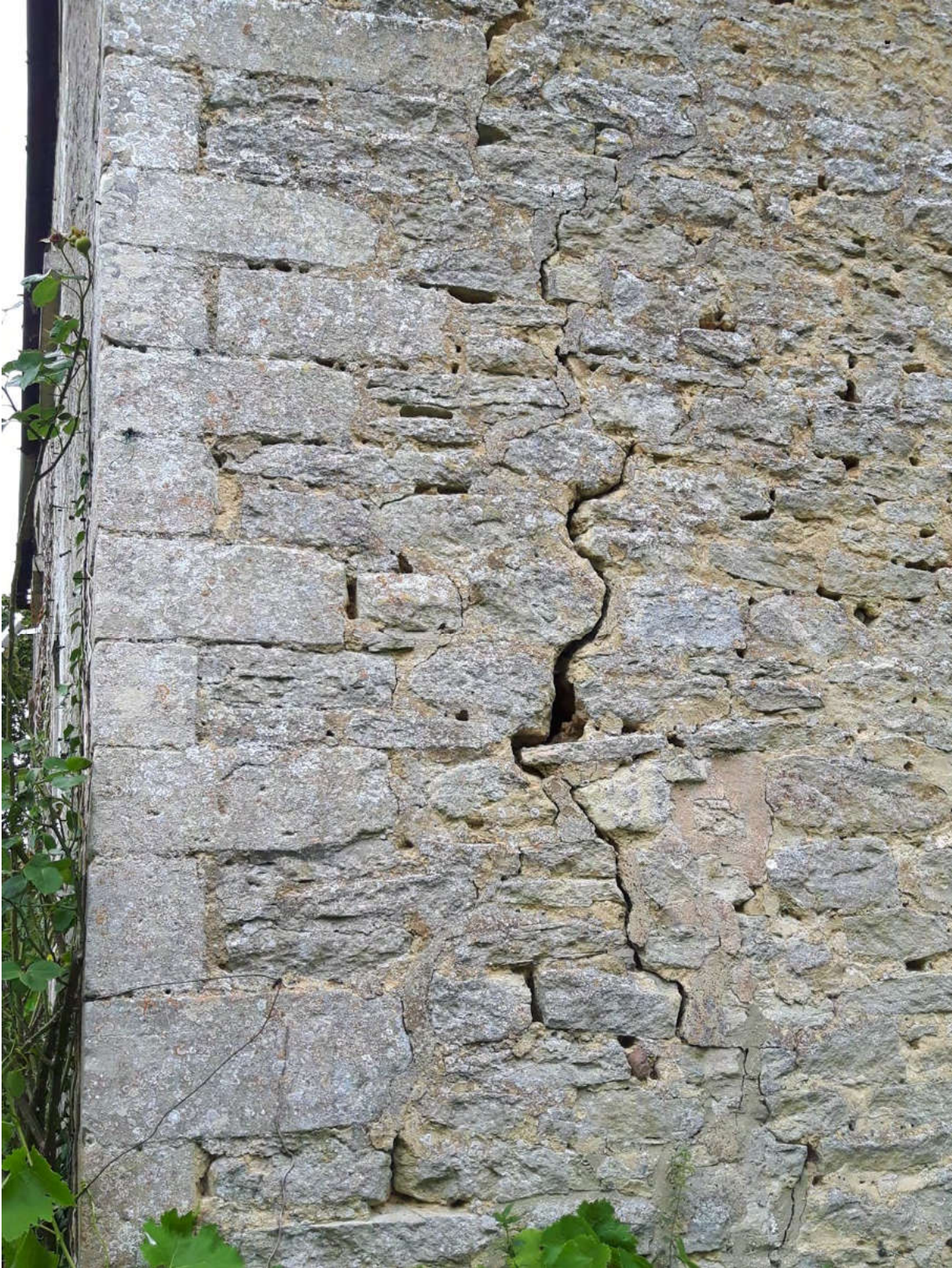
Photograph 2 - Cracking to east wall indicating relative movement with south wall
