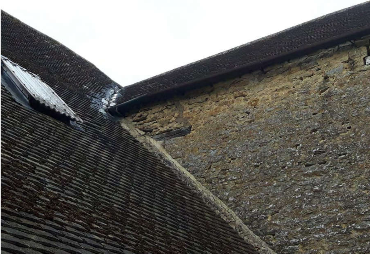
Photograph 16 - Junction between roofs with previous repair and embedded timber
