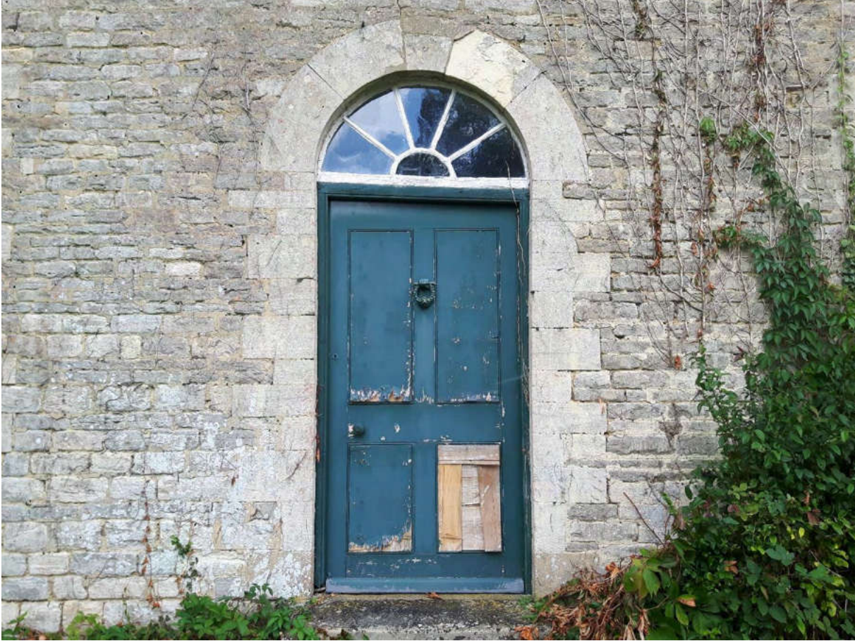
Photograph 4 - Differential movement through arch lintel
