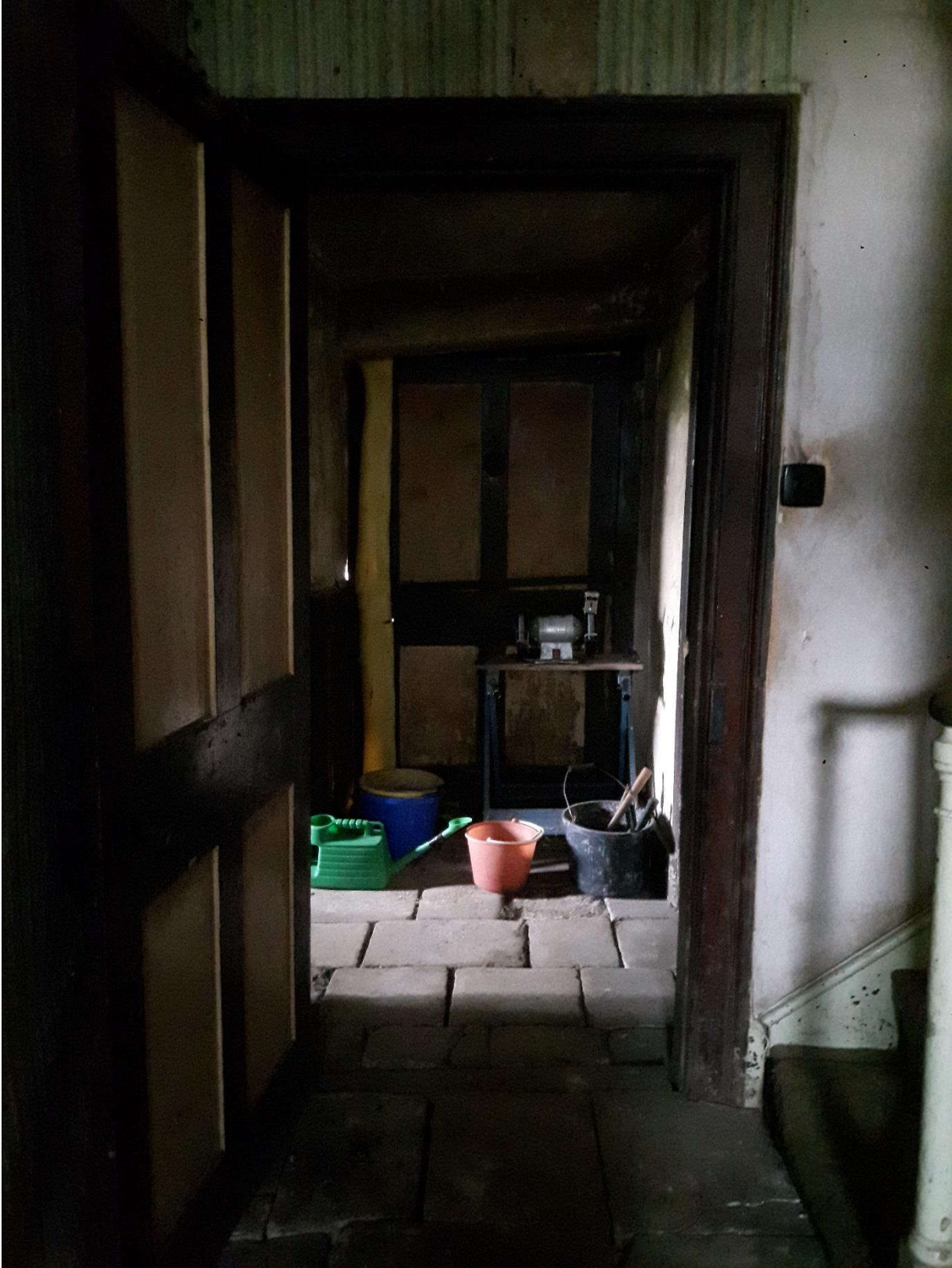
Photograph 8 - Main hallway floor relative to north door lintel
