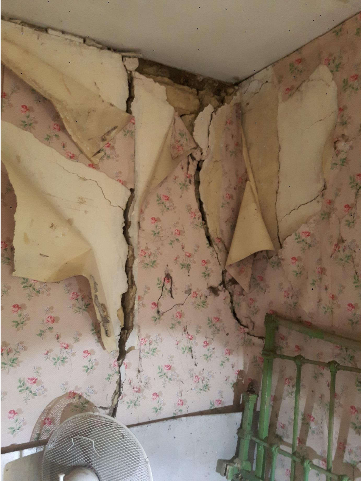
Photograph 12 - Severe cracking in first floor spine wall and separation from west wall
