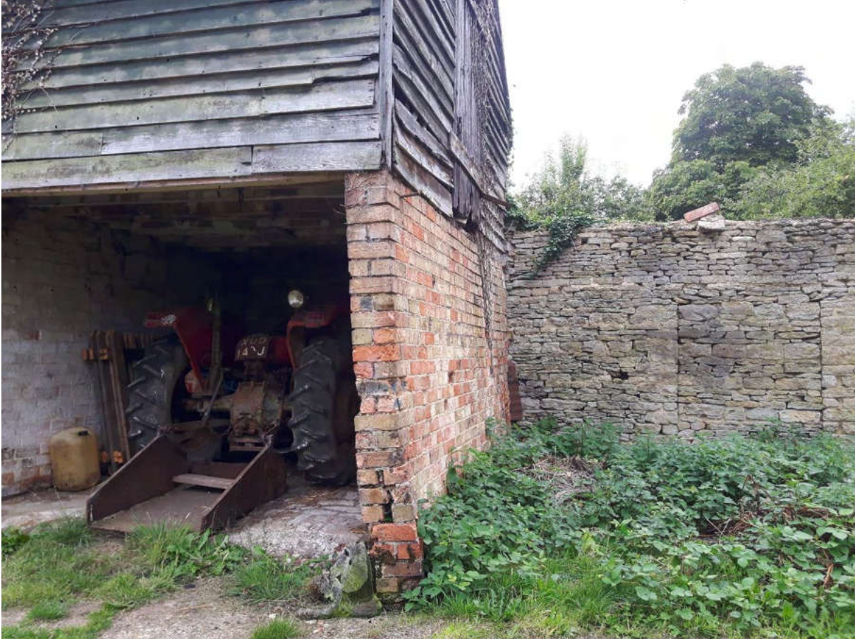
Photograph 18 - Block A, leaning wall and tree stump
