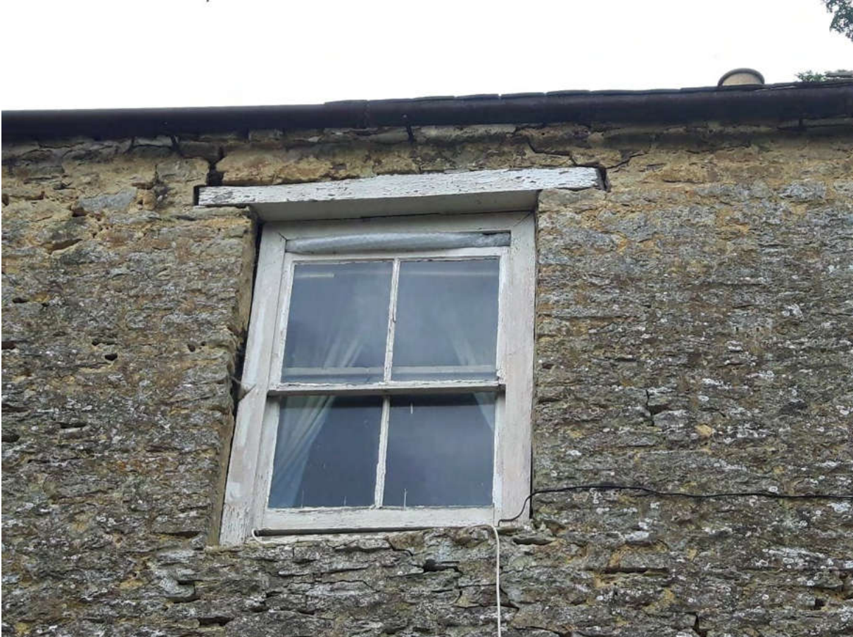
Photograph 7 - Movement and cracking around timber lintel
