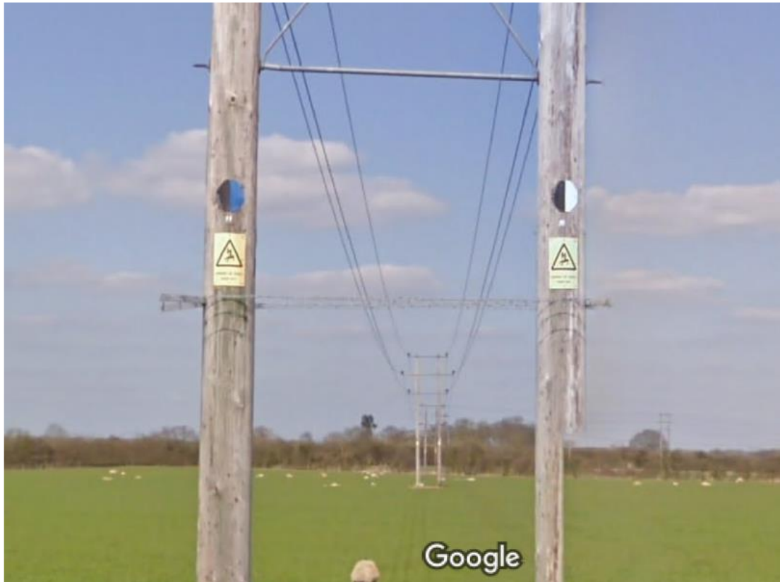
Figure 4: Bicester – Headington 33kV feeders' courtesy of Google maps
