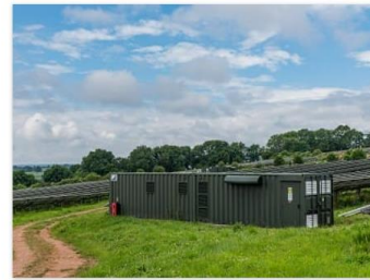
Coleford Solar Farm Inverter-Transformer Station
