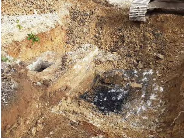
25.04.22 – Removal of soils around interceptor prior to breaking out. Black stained soils visible in base of excavation
