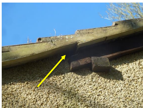
Photo 14: Potential bat access at eastern elevation
