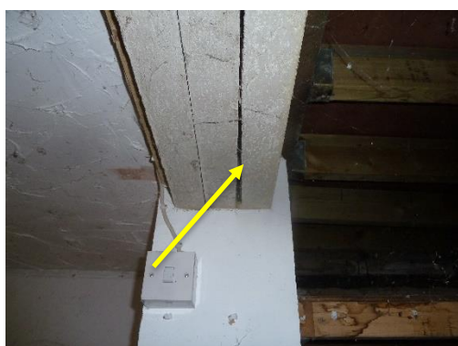
Photo 16: Gap in lintel by lean-to, full of cobwebs
