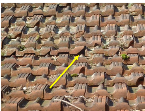
Photo 15: Potential bat access point under tiles
