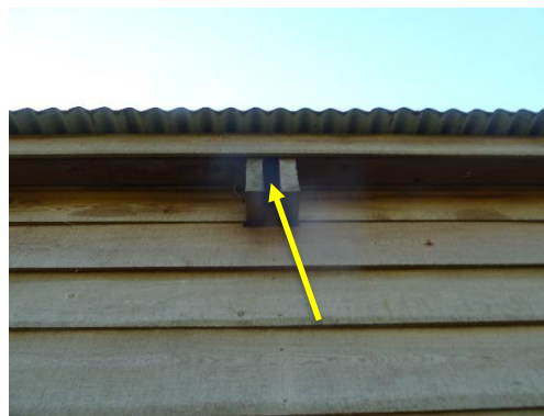
Photo 7: Potential bat access to interior of building 3
