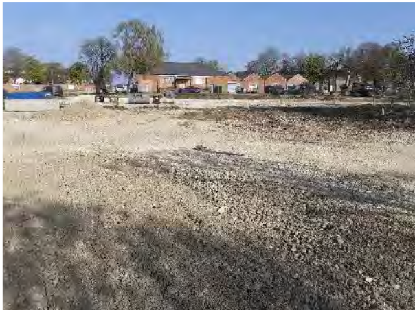
20.04.21 – Western view across the site with exposed natural soils present following hardstanding removal.
