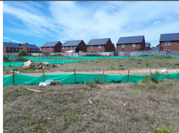
02.06.20 – Site surface occupied by light vegetation. Ecological fencing up during on-going survey work
