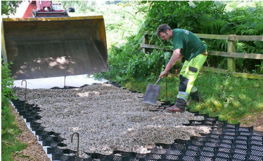
Figure 1. Example of no-dig footpath construction using a cellular confinement system laid on-top of existing round levels.
