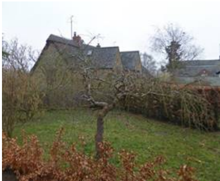
Nos 2 and 3 each have a rear gable extension with pitched roofs dating from 1981. The southern wall of the extension at No 2 forms the boundary between Nos 1 and 2.
