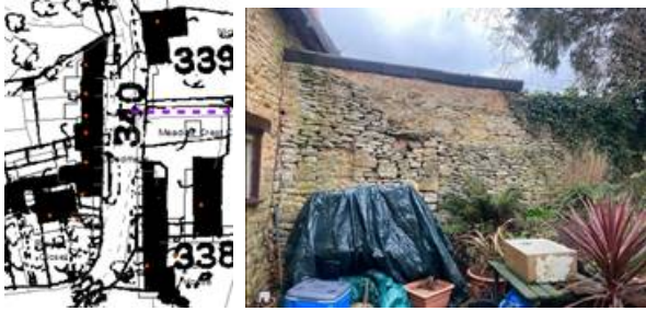
1875-87 OS Map and the boundary wall with Goodmays showing the scar of the former small single-storey lean-to. The wall to the extension at Goodmays has increased the height of the boundary wall.
