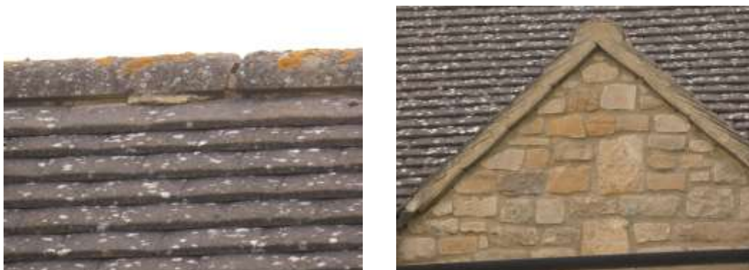
Figs. 7 & 8 Mortar crumbling at the ridge but verge fully pointed
