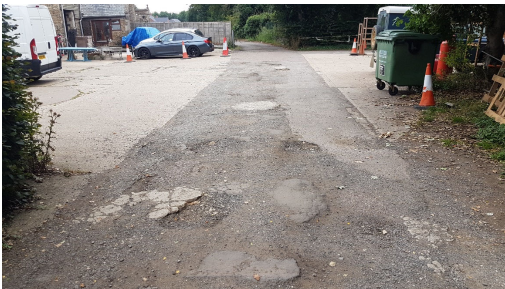
Photo 3: View of shared access and concrete hardstanding looking west towards the subject site
