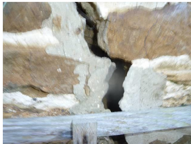
Crack in stone wall of single storey element
