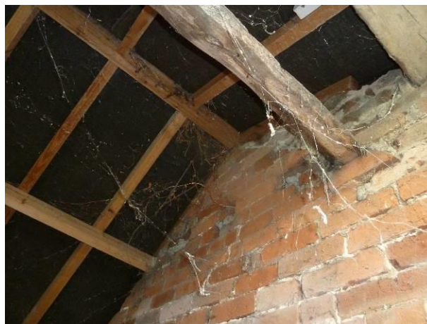
Cobwebs in single storey element
