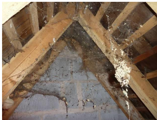
Cobwebs in Void A
