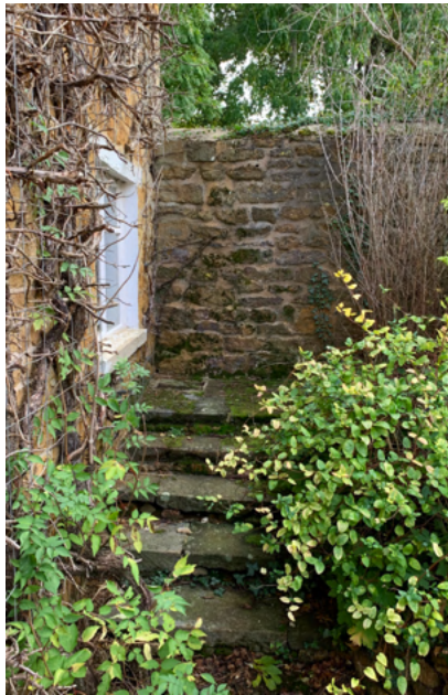
Fig. 29, Steps leading from the front of the house beneath the later eastern boundary wall.
