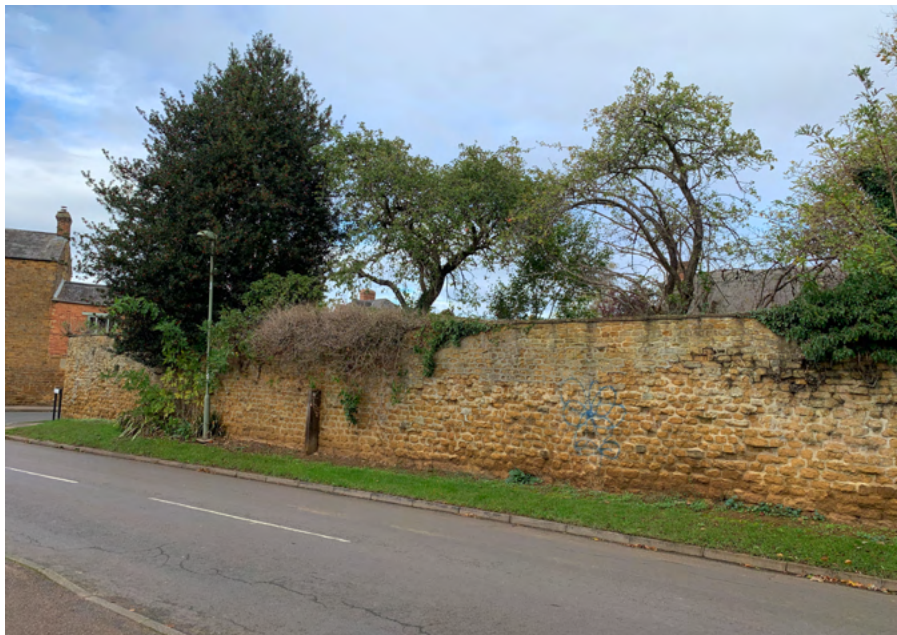
Fig. 30, The boundary wall on Broad Gap, where the proposal is to create new vehicle access, approximately where the graffiti is. This could be mitigated by the insertion of tall gates.
