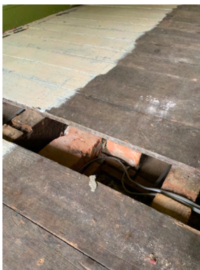
Fig. 14, The upper part of the dining room/kitchen partition exposed beneath the boards in bedroom 4.
