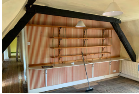
Fig. 17, Bedroom 1 roof truss. Note how the truss blocks the existing entrance to the room. The partition behind is proposed for removal, relocated to this side of the truss.
