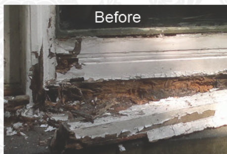
Rotten unsalvageable sill
