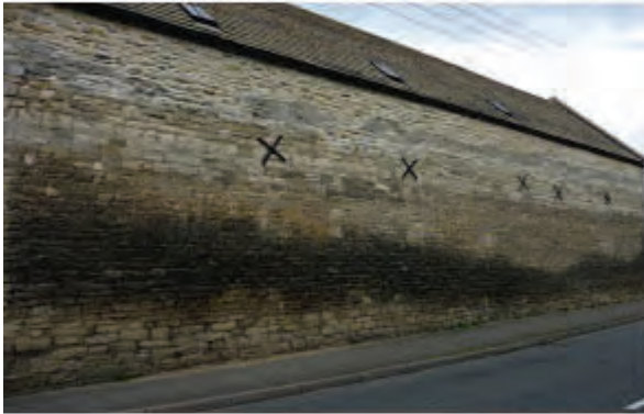
Soiling of The Dashwood Arms accommodation block by road spray.
