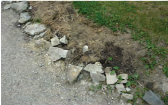
Erosion of kerbing
