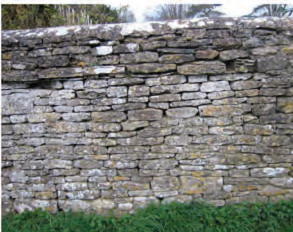
Heaped mortar forms coping
