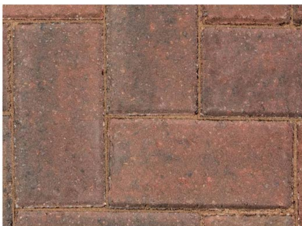
02 027 BLOCK PAVING TO PATHS brindle
