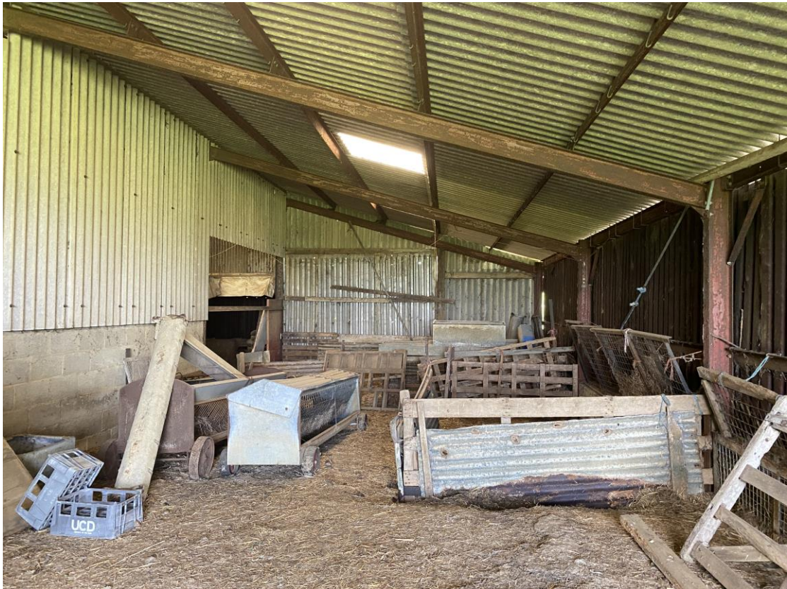
Eastern lean to. Mid height cladding rail to Eastern elevation to be modified in 3 bays.
