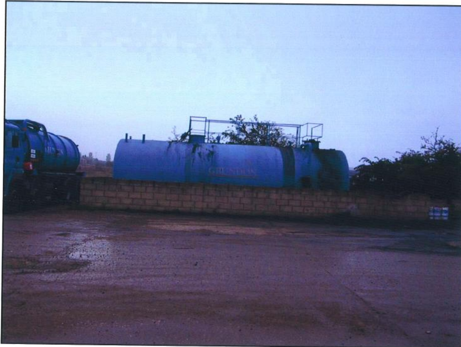
Plate 5: Oil storage in Grundon compound.
