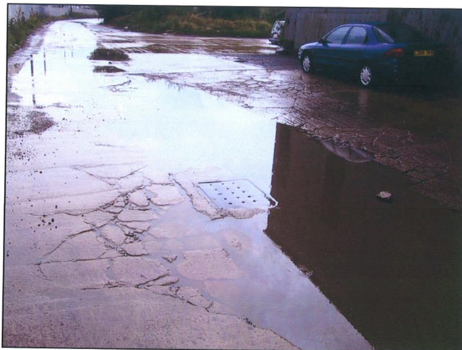
Plate 10: Collapsed drain outside Friswell Blackbushe.
