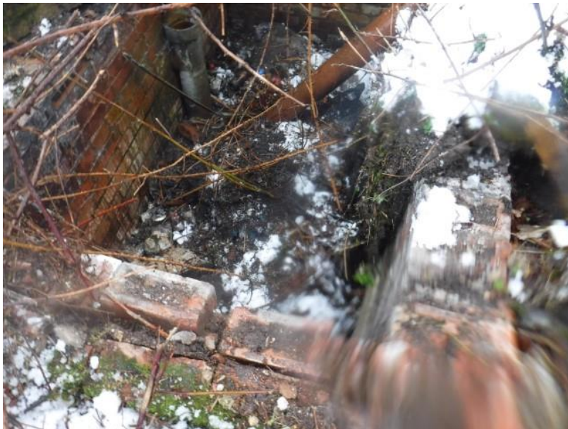
Sceptic Tank Housing
