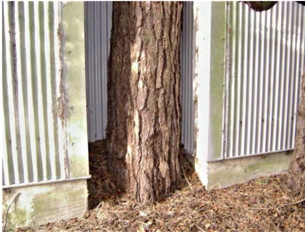
Photograph 13 – Pine tree T76 with the stem enclosed on three sides by the concrete base of the building.
