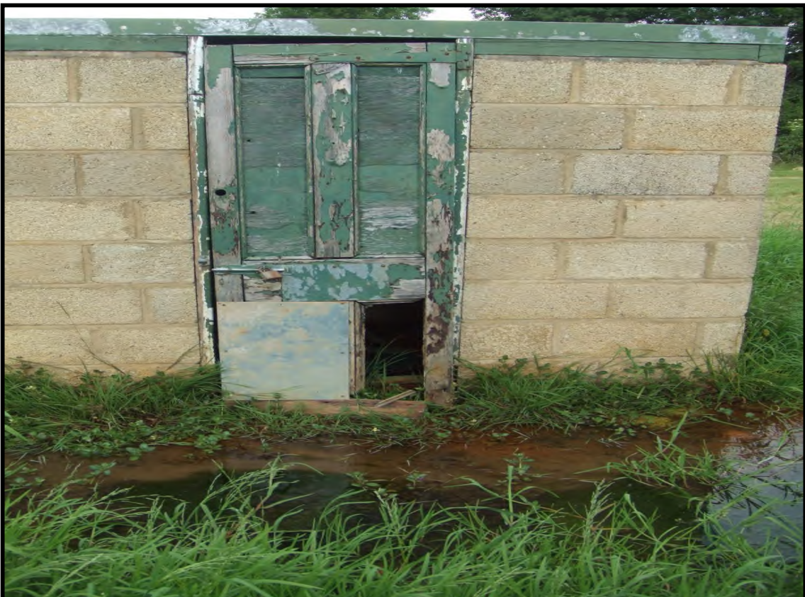
Plate 10: Water Abstraction Point located on Messrs. Malins' land, between two mobile telecommunications masts (see Reference B3 on the Envirocheck Information drawing in Appendix A)
