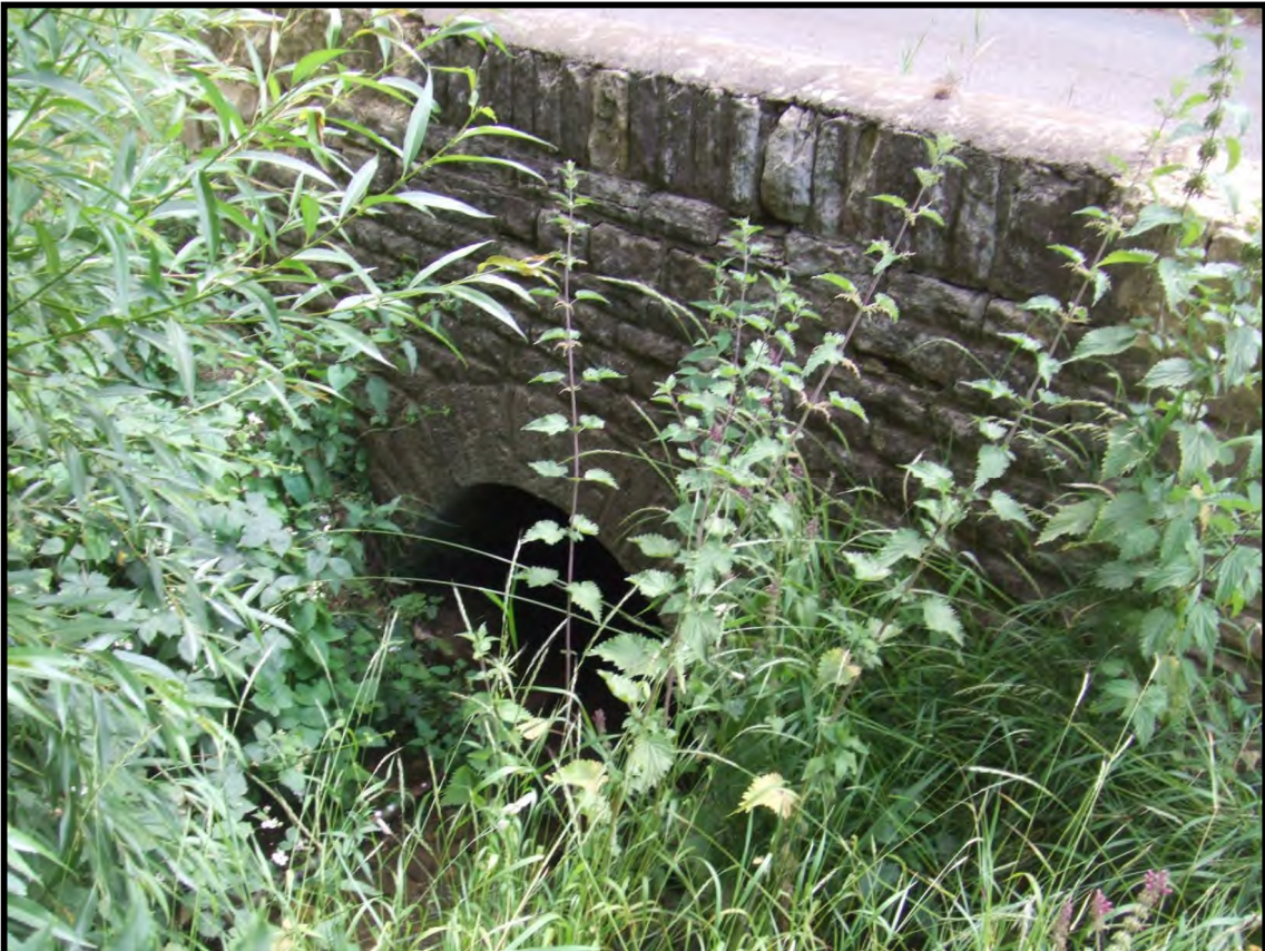
Plate 3: Stone-faced drainage culvert crossing beneath Bucknell Road at a location some 500m NW of the junction (roundabout) with the A4095 (Lord's Lane)
