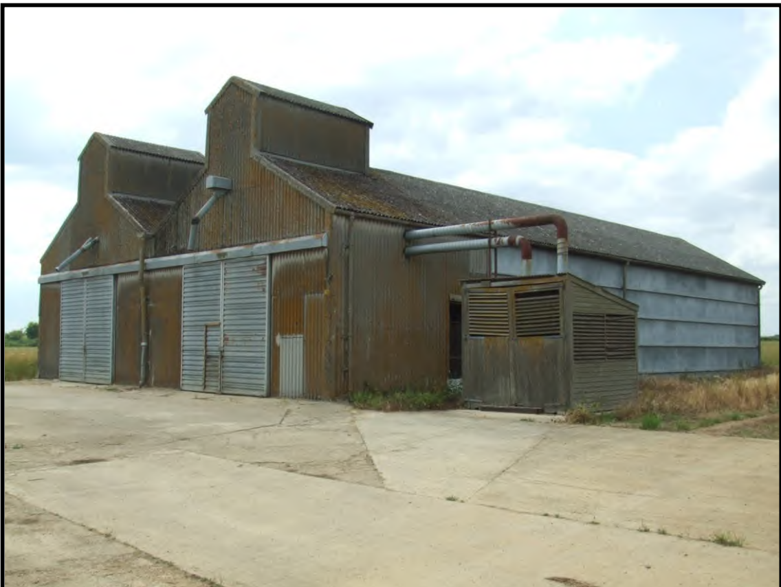
Plate 4: Asbestos clad building along Bucknell Road, located some 950m NW of the junction (roundabout) with the A4095 (Lord's Lane)
