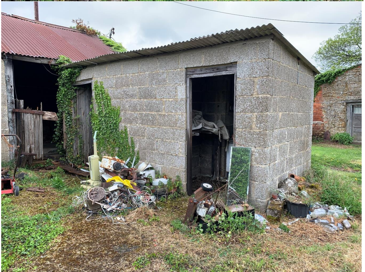
Figure 16: Building 6 (top) looking south-east, and buildings 7 and 8 looking north-west. The former's condition has deteriorated since 2016 – compare with the same view in Soden 2016, figure 12.
