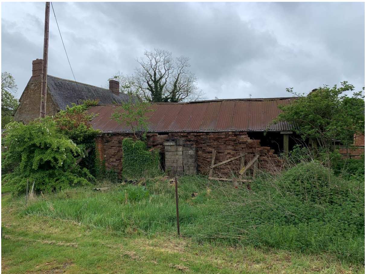
Figure 17: Buildings 7 and 8 looking south-east (top), and the rear wall of buildings 7, which is in very poor condition.
