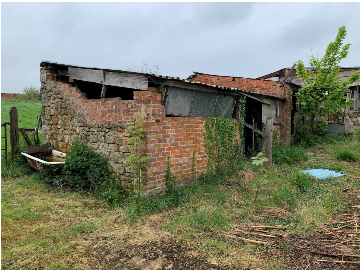
Figure 15: Building 5 looking north-west. The ironstone end wall may be of 19 th -century date. All the rest is modern. Including the roofs.
