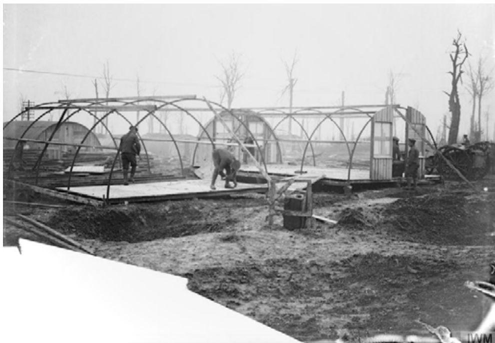
Fig 8: British troops erecting Nissen Huts during WW1. The huts would become quite ubiquitous during the Second World War due to their ease of construction. ©IWM
