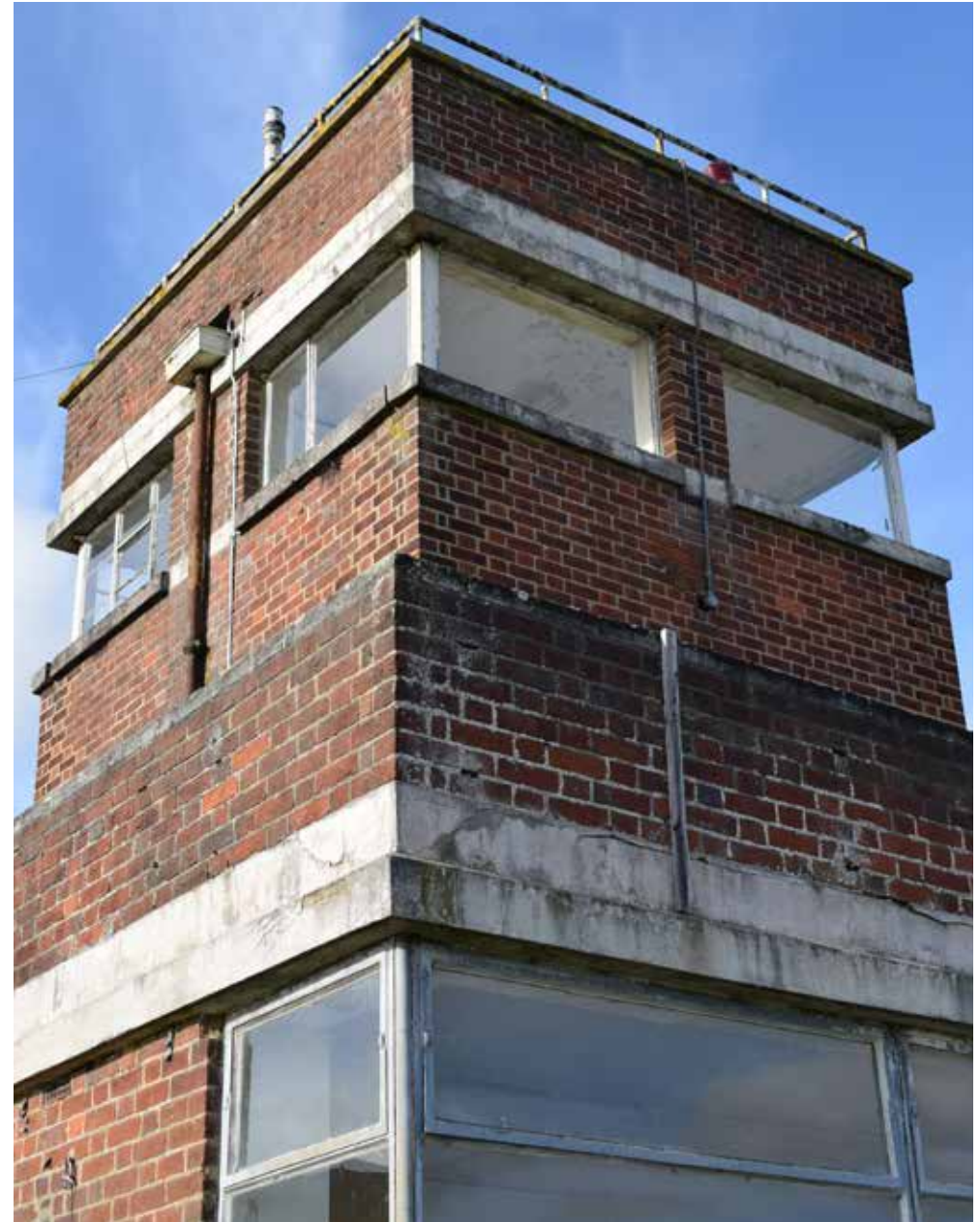
Fig 52: Detail of the watch tower, designed to allow surveillance over the entirety of the flying field
