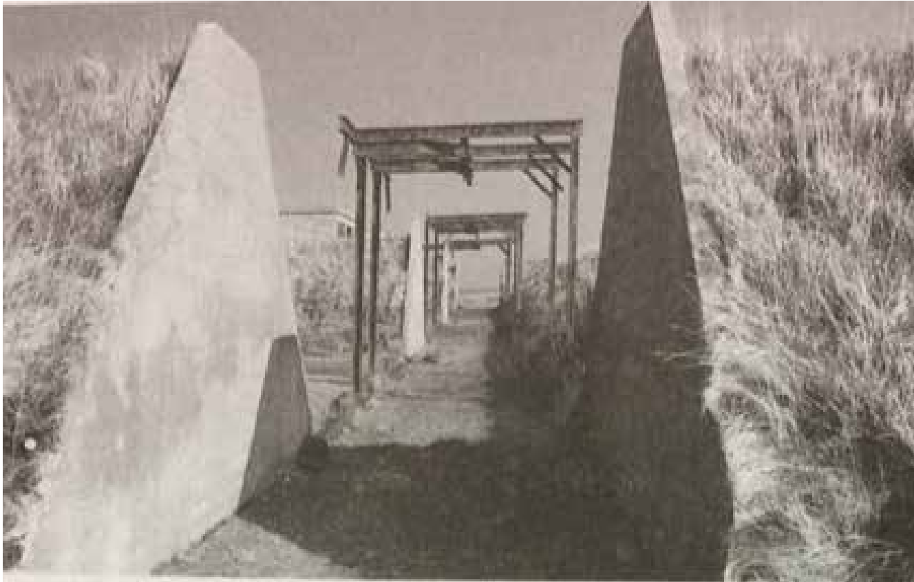
Fig 15: Bomb store area at RAF Wick. Showing the earth traverse walls and the surviving steel frame structure for the bomb hoisting cranes (Francis 1996: 42)
