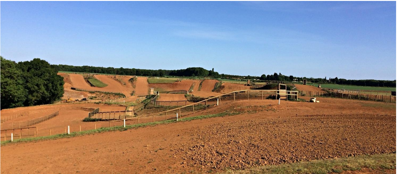
Above: After further earthworks during Covid lockdown, May 2020 (Photos this page: Hornton villager)
