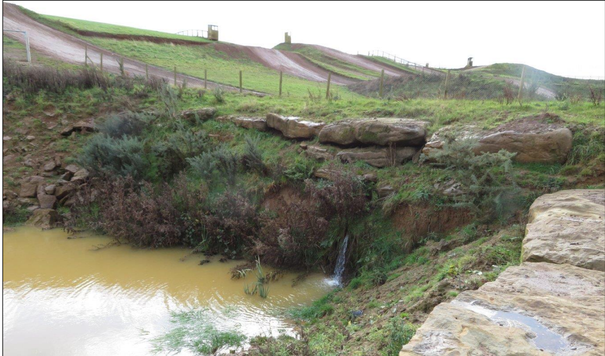
Figure 14 The western end of the upper pond shows inflow from the south
