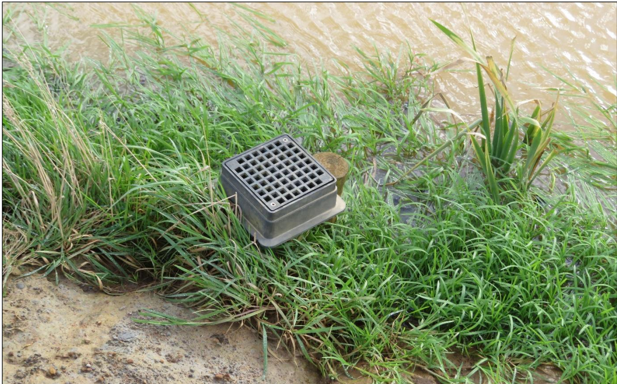
Figure 16 Overflow from the upper pond, installed as a precaution against blockage or exceedance of the outflow
