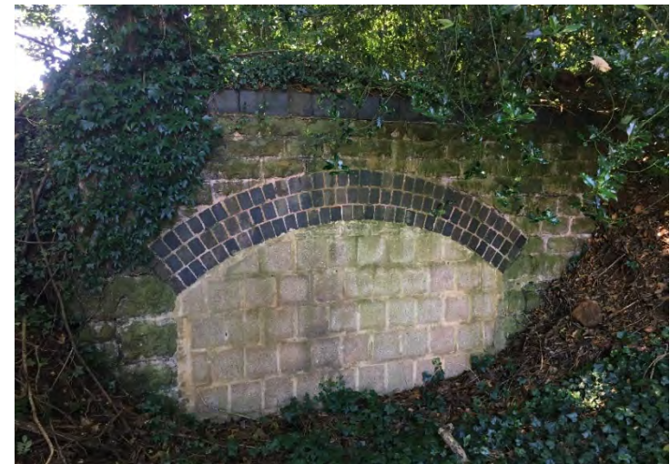
Plate 8: Close-up of infilled subway arch in the south-western corner of the site
