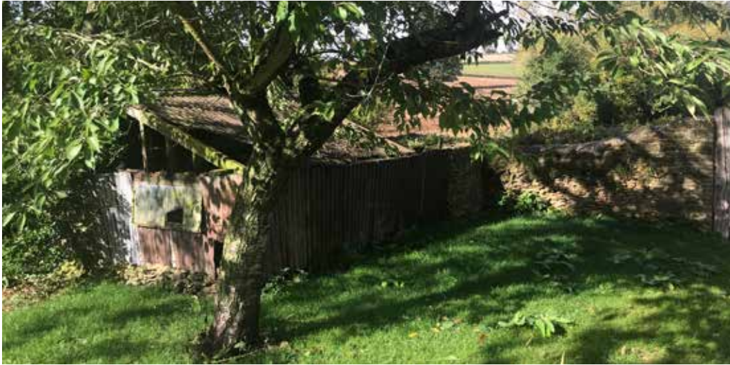
View of the dilapidated log store
