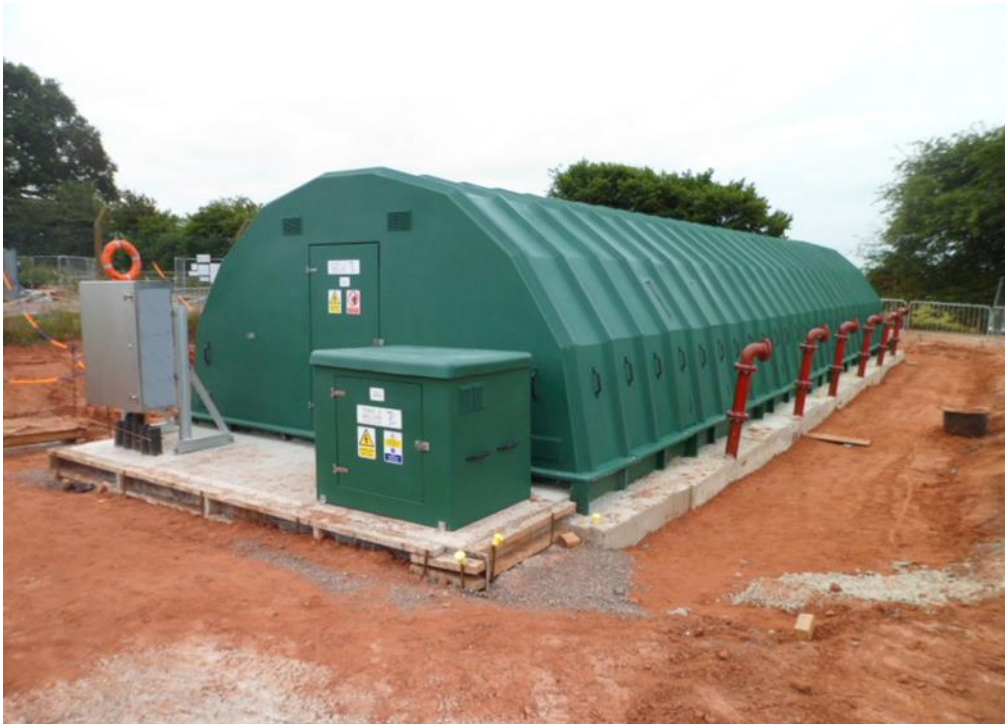
Typical RBC installation nearing completion with front apron (Heyford RBC will not have the small green compressor kiosk)
