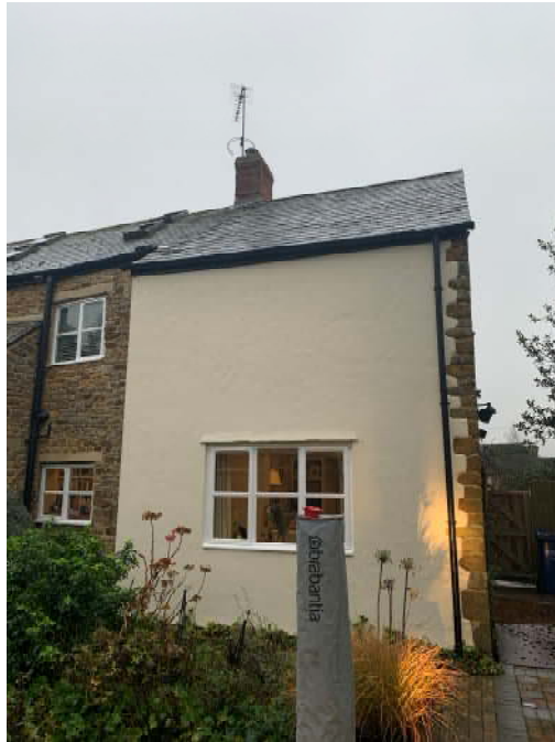
Northern elevation showing plaster render fascia board and guttering and slate covered roof.
