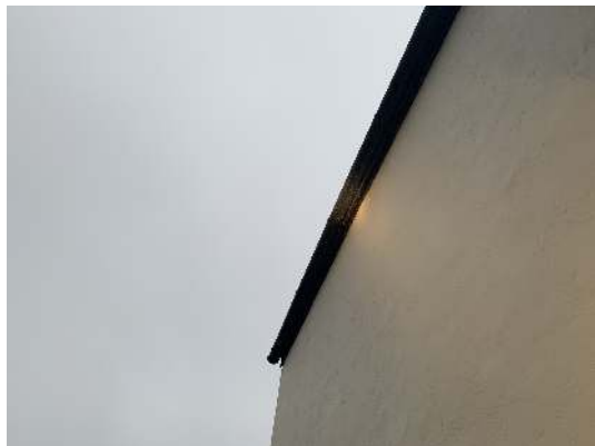
Northern elevation showing fascia board and guttering. Grey marks on guttering are the sucker stains left by Virginia creeper.
