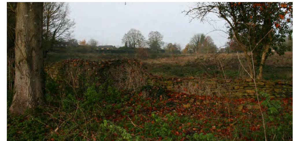
Existing stone wall along southern boundary to be repaired
