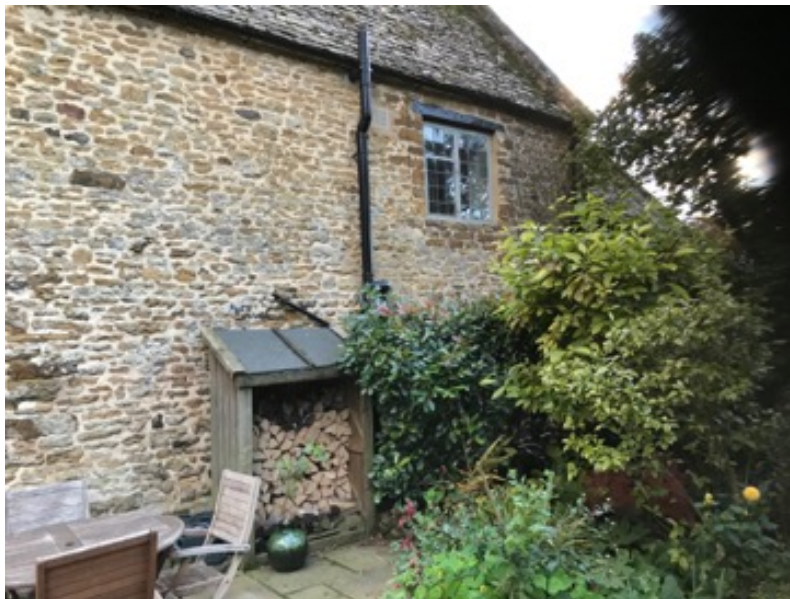
View of the north elevation of Stickley House from the garden of Pond Cottage, both the ground and first floor windows on this elevation are modern
