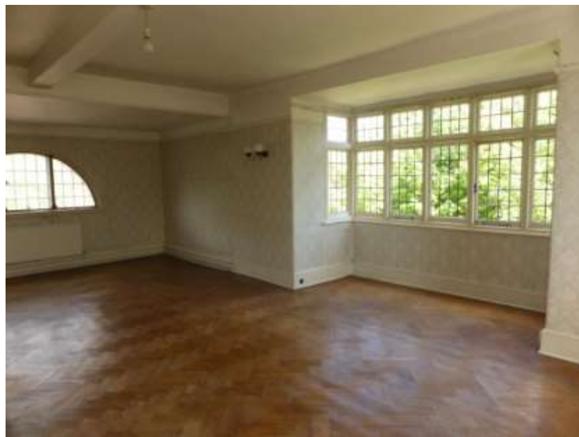
Figure 49: Re-set thermal window to the left and early 20 th century oriel to the right
