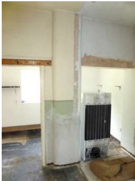
Figure 32: Plaster finish over a brick pier in G7
