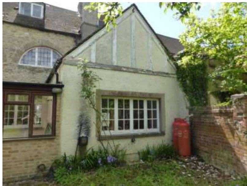
Figure 18: Early 20 th century single storey extension on the right hand side of the rear elevation
