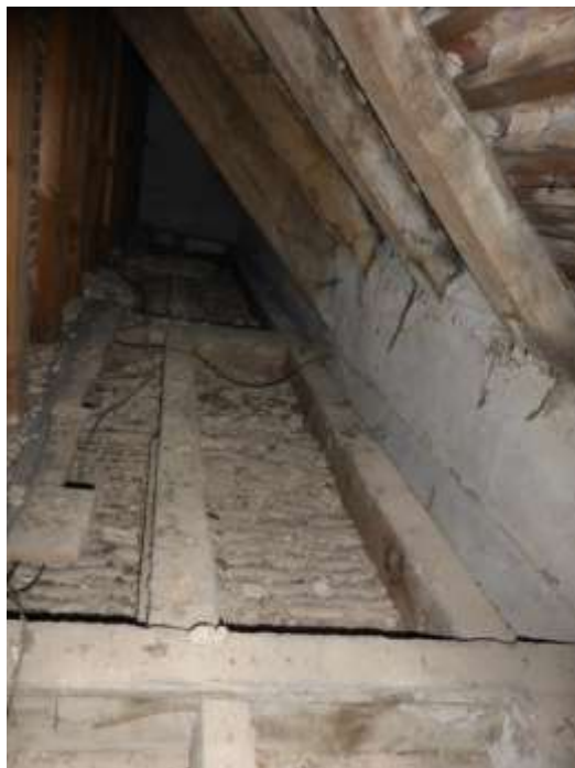
Figure 58: Structure of the ceiling over F5 and machine sawn timbers of an ashlar wall in A5
