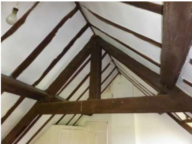
Figure 57: Machine sawn collar and king post in A5
