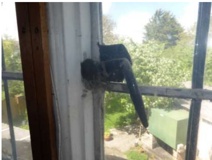
Figure 52: Detail of L-shaped bar catch to the casement of the thermal window in F5
