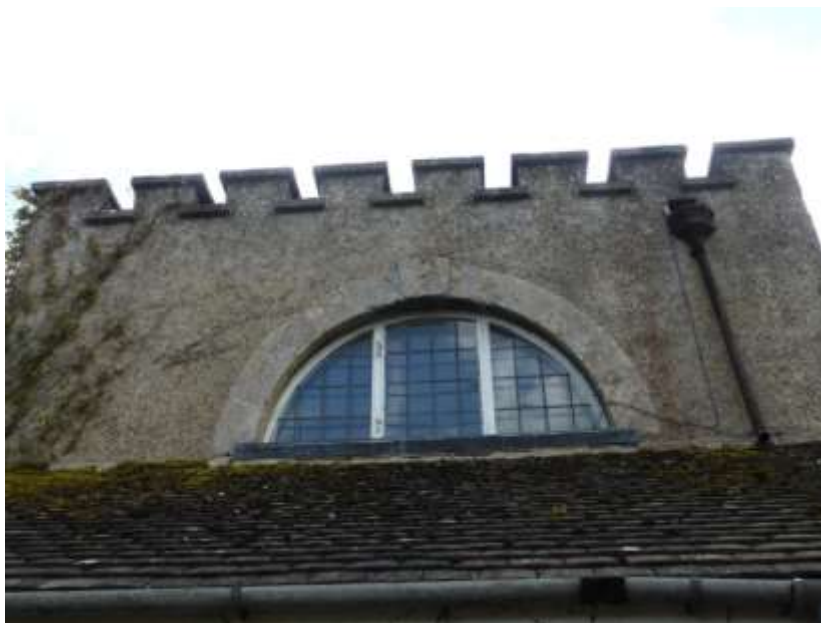
Figure 16: Repositioned thermal window on the north elevation of the early 20 th century crenelated extension
