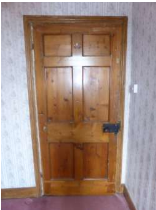
Figure 40: Probable early 20 th century door to F1
