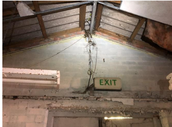
2. Small area of remaining ceiling
