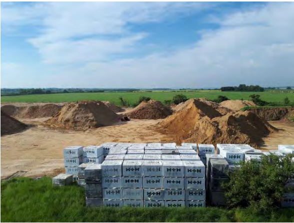
22.05.18 – Temporary stockpile storage area in the south. Development arisings generated from wider Heyford development
