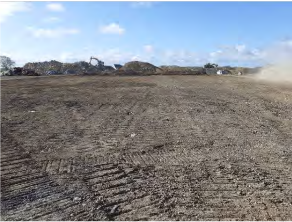
06.04.21 – Western part of site demolition complete, hardstanding removed, and site regraded ahead of formation sampling
