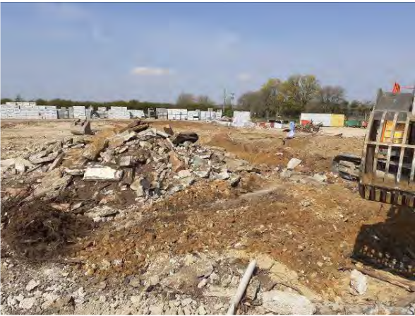
20.04.21 – Handpicking of ACM fragments within localised area in the north (HS-ACM) by specialist sub-contractor
