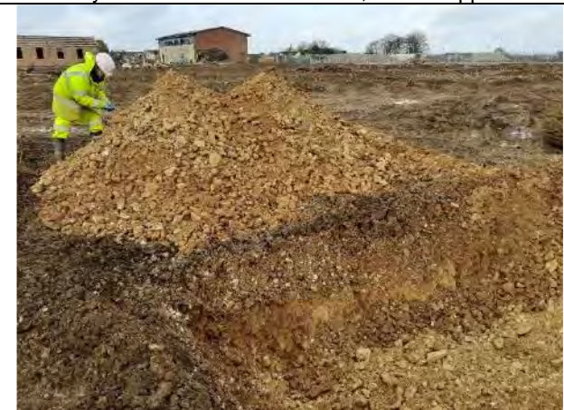
17.02.21 – Inspection of arisings and collection of validation samples. No visual or olfactory evidence of contamination, PID <0.1ppm.
