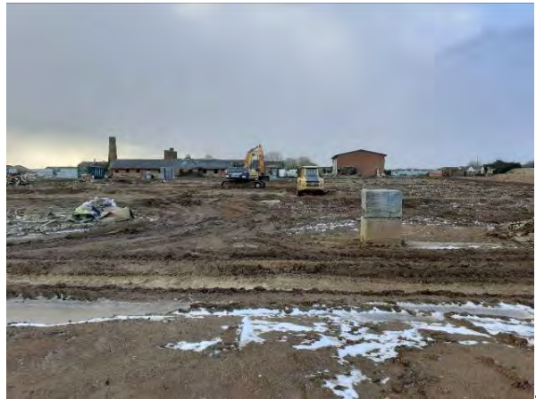
08.02.21 – Easternmost line of building demolished and hardstanding removal prior to surface level regrade
