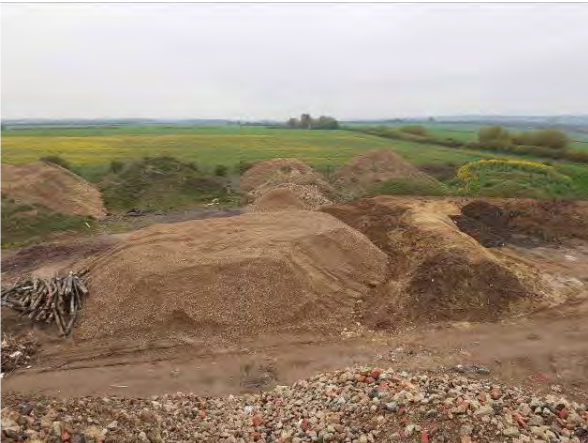
28.04.21 – Stockpiles of arisings generated from wider Heyford development temporarily stored in the south
