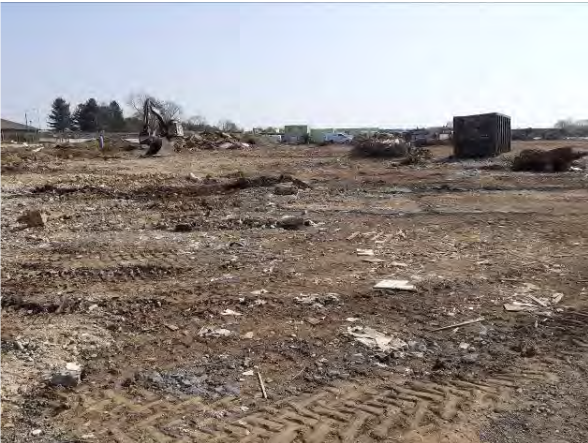
20.04.21 – Eastern view across the north of the site following building demolition and hardstanding removal but prior to regrade
