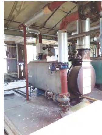
22.05.18 – boilers within boiler house
