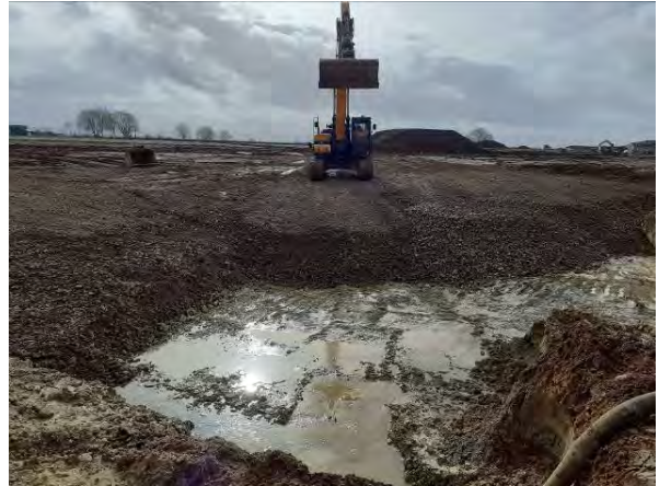
17.02.21 - Backfill of remediation excavation immediately following the collection of samples due to the ingress of groundwater
