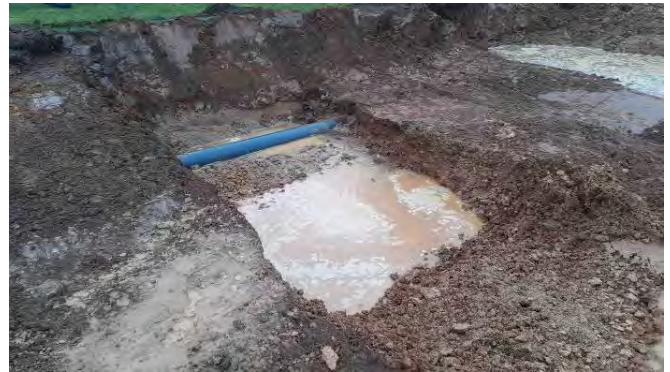
14.01.21 – Exposure of POL pipeline in the north. Shallow ingress of groundwater, no sheen, floating product or globules observed.
