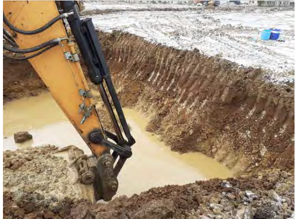
08.02.21 – Recovery of clean overlying soils from hotspot area. Ingress of shallow groundwater, no sheen, globules or floating product observed.
