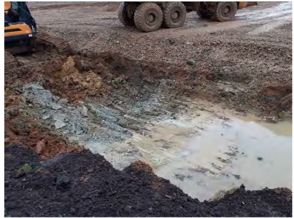
18.02.21 – Removal of impacted soils down to layer of clean clay above shallow bedrock
