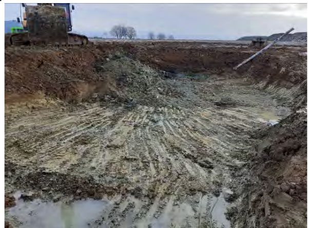
09.02.21 – Removal of impacted soils until visual, olfactory indicators absent and low (<10ppm) readings recorded on PID. Base of excavation in northeast onto clay.
