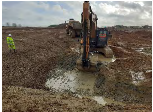
16.02.21 – Removal of impacted soils down to bedrock. Ingress of groundwater at surface of bedrock, no sheens observed.
