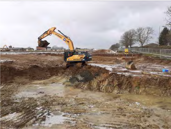
10.02.21 - Recovery of clean surface soils to allow removal of underlying impacted soils.
