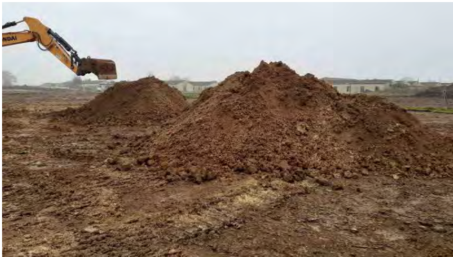
14.01.21 – Clean soils temporary stockpiled on surface to allow inspection prior to relocation to temporary holding area
