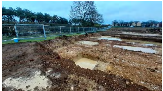
14.01.21 – Eastern view across the hotspot area with partial recovery of clean surface soils and a series of trial-pits / trenches to delineate extent
