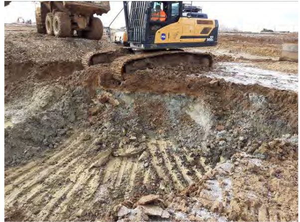
10.02.21 – Light grey soils below light brown visible denote fuel impacted soils.
