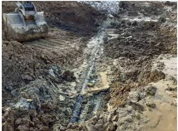
09.02.21 – Exposure of POL pipeline which ran north to south through the centre of the baseball pitch
