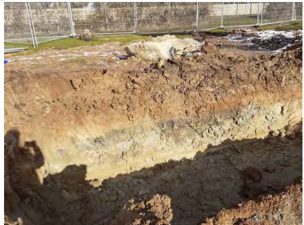
09.02.21 – Northern sidewall of remediation excavation absent of any significant contamination indicators suggesting sufficient removal of impacted soils
