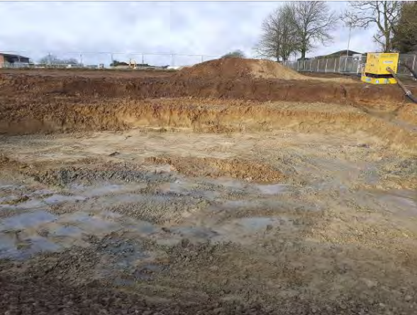
17.02.21 - Completed extent of remediation excavation in the north / northwest. Base and sidewalls ready for validation samples to be collected
