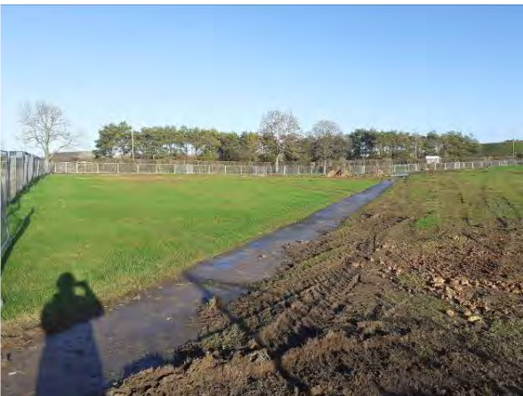
15.12.20 – Northeast view across path which crosses the western end of the site
