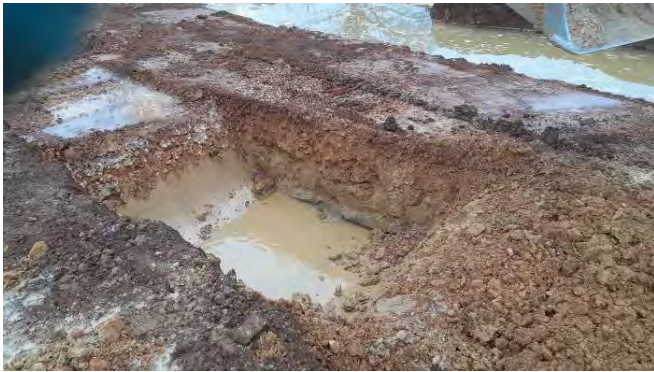
14.01.21 – Excavation of a series of shallow trial-pits to delineate extent of impacted soils
