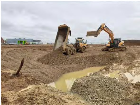
16.02.21 – Backfilling of remediation excavation with aggregate concurrently with removal of impacted soils
