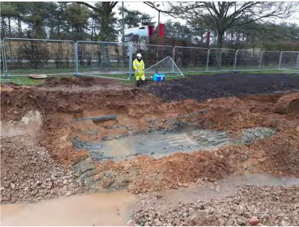
18.02.21 – Grey impacted soils awaiting removal following removal of clean overburden. Pipework in sidewall drainage pipe and not POL pipeline
