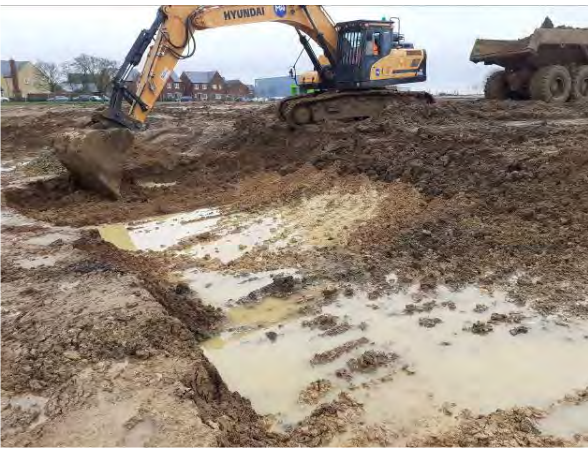
02.02.21 – Excavation of clean overlying soils and removal from remediation area to allow extension down to impacted soils
