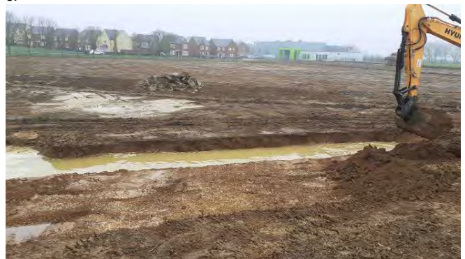
14.01.21 – Stripping and recovery of topsoil complete. Trenching to delineate extent of impacted area to allow initial recover of clean overburden soils
