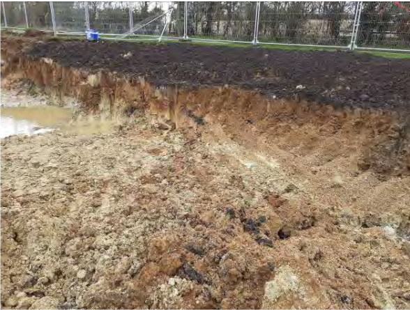
18.02.21 – Northern extent of remediation excavation due to the presence of trees with protection orders
