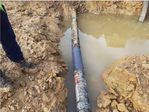
03.02.21 – POL pipeline exposed in the northwest. Wrapping around pipework suggests possible historical repair work
