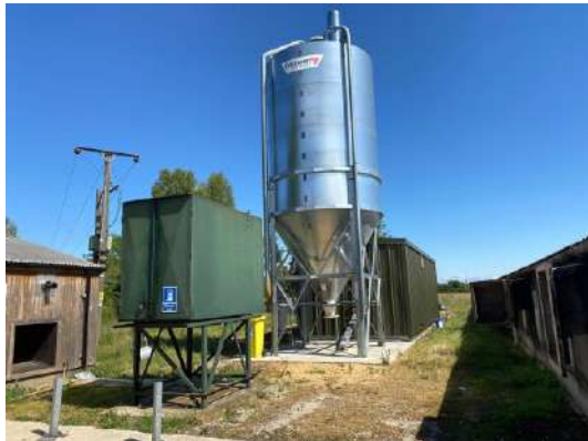
Above ground diesel tank in the west of the former chicken farm, view facing north.
