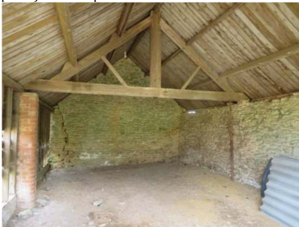
Photograph 7. The interior of the northern end of the western part of the L-shaped barn (Figure 3: A1)
