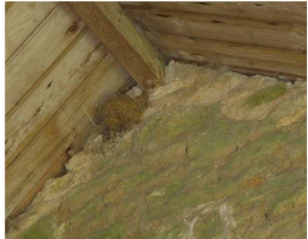
Photograph 34. Swallow's nest in the central section of the western part of the L-shaped barn (Figure 3: A2)
