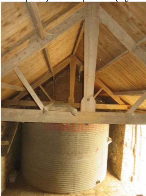
Photograph 9. The interior of the southern end of the western part of the L-shaped barn (Figure 3: A3)
