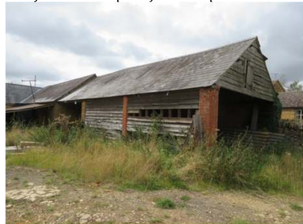
Photograph 4. The north and east elevations of the northern end of the western part of the L-shaped barn
