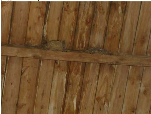
Photograph 35. Swallow's nest in the western section of the southern part of the L-shaped barn (Figure 3: A5)
