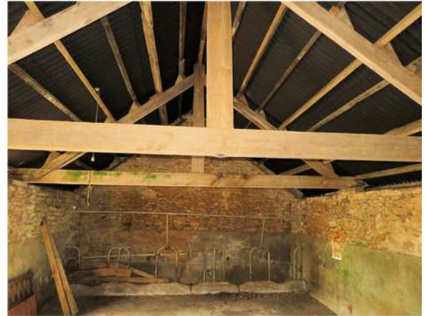
Photograph 12. The interior of the eastern end of the southern part of the L-shaped barn (Figure 3: A6)
