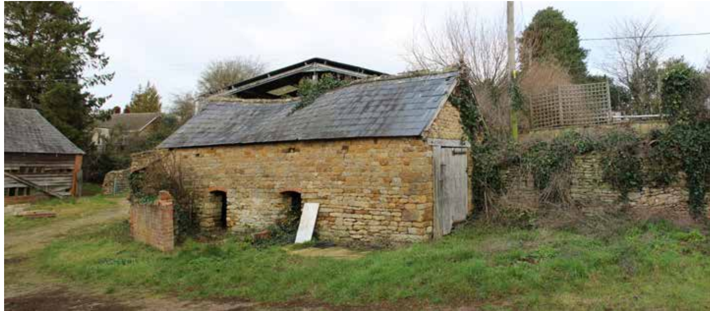
View 16 - View of piggery looking north with the upper level garden to the right
