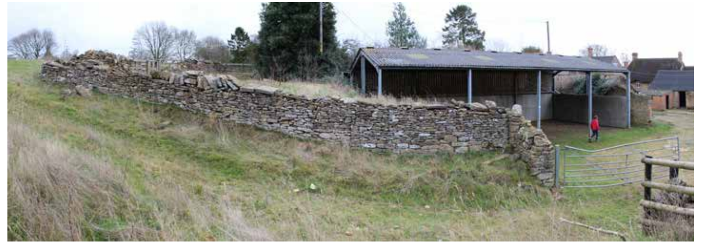
View 22 - Looking east from the access track towards the boundary wall and modern steel barn structure
