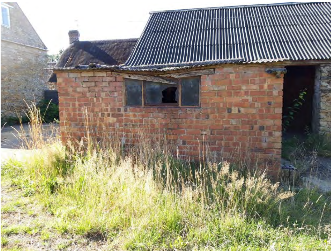
Photograph D: Looking south at brick building attached to the L-shaped building
