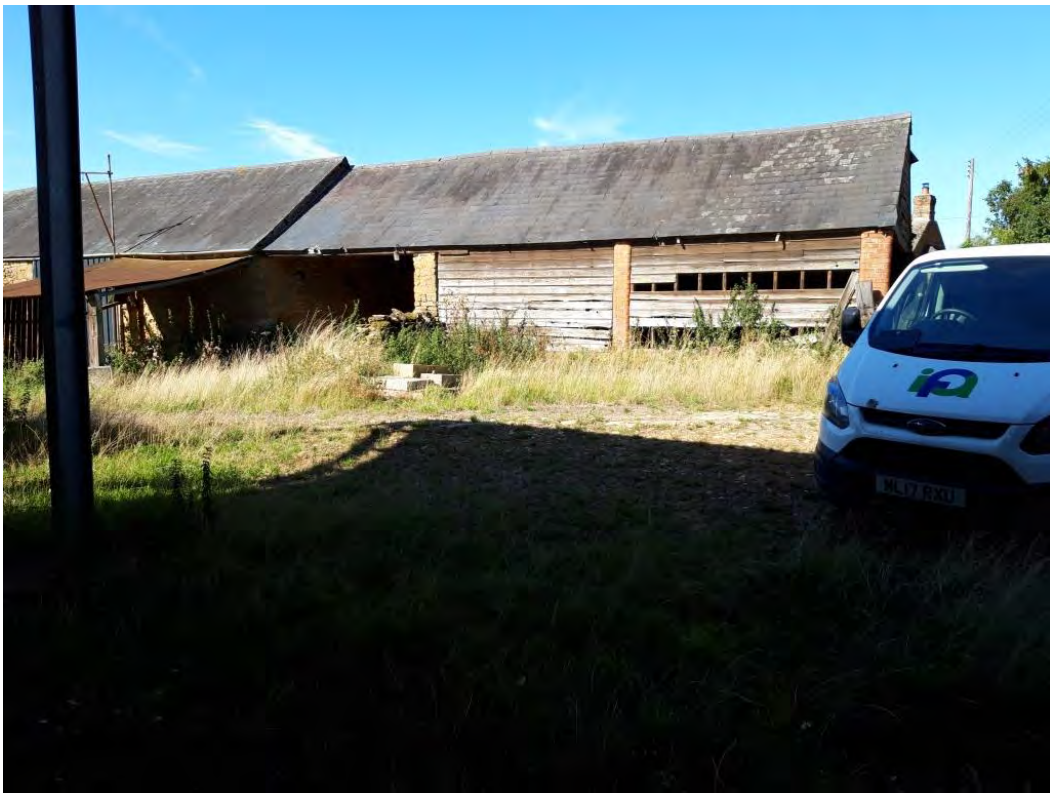
Photograph B: Looking west at the open end of the L shaped building
