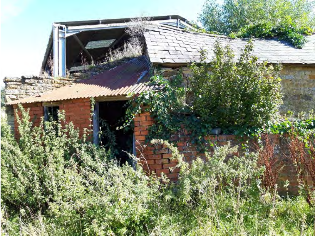
Photograph G: Looking northeast at the piggyery and bulging brick wall with modern storage barn beyond
