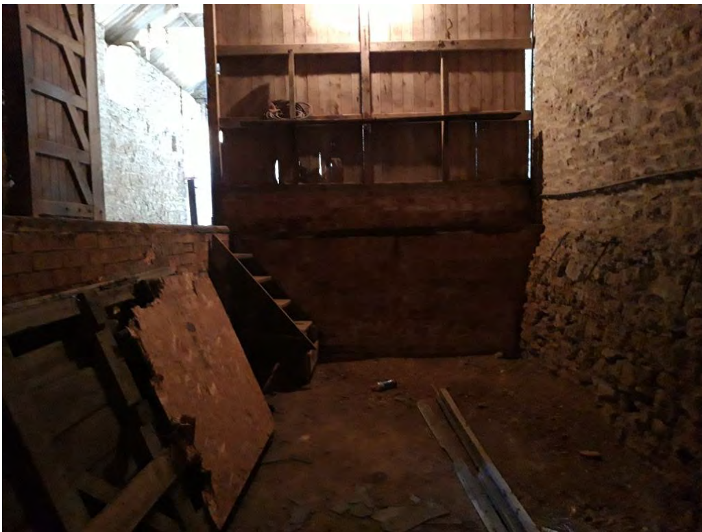
Photograph F: Looking west from the southwest corner of the site within the lower ground loading bay
