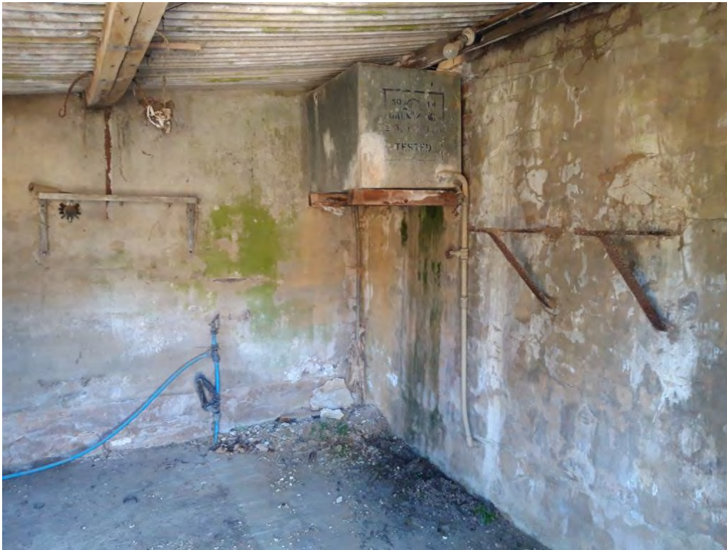
Photograph E: Internal view of the brick building including a suspected water tank
