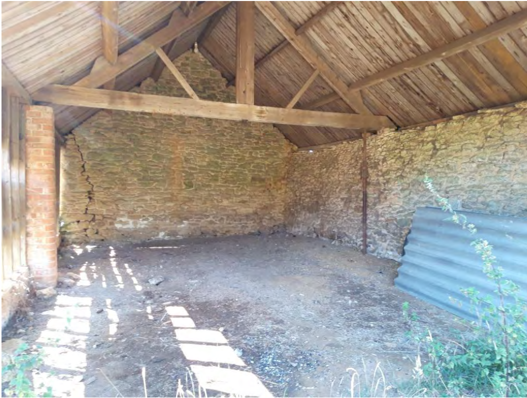
Photograph I: Looking south at the crack present within the open end of the L shaped building
