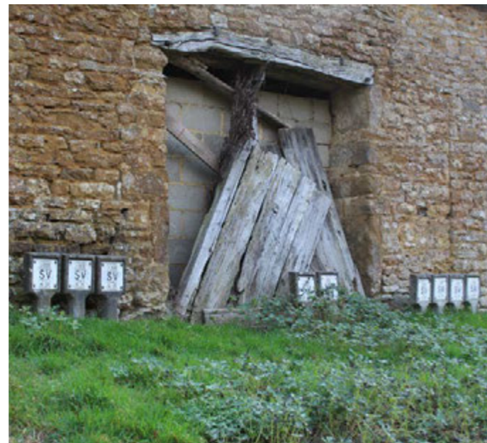
Fig. 27 - Inappropriate and substandard repairs
