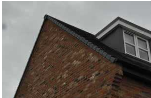
Inappropriate use of upvc clip edges, and fascias to gable
