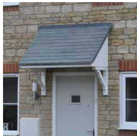
Unsuccessful example of plastic faux-tile porch, Banbury
