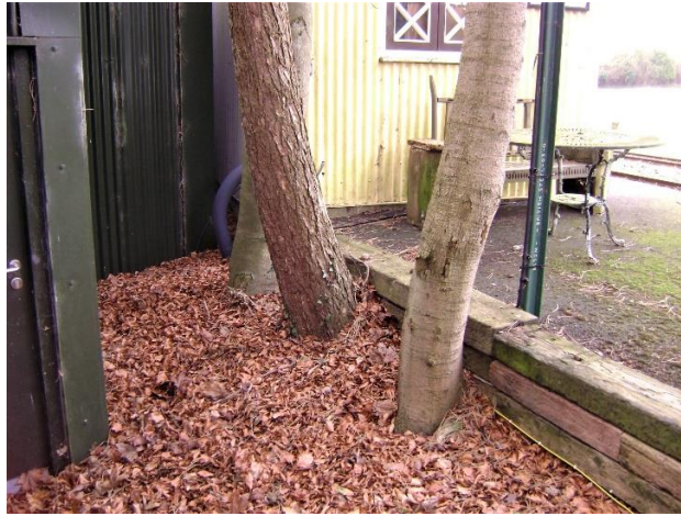
Photograph 12 – The base of Maple tree T70, Larch tree T71 and Beech tree T72 at the back of the raised platform.
