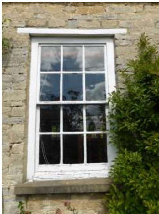
Figure 5: Ground floor six over six sash window with timber lintel and rendered sill
