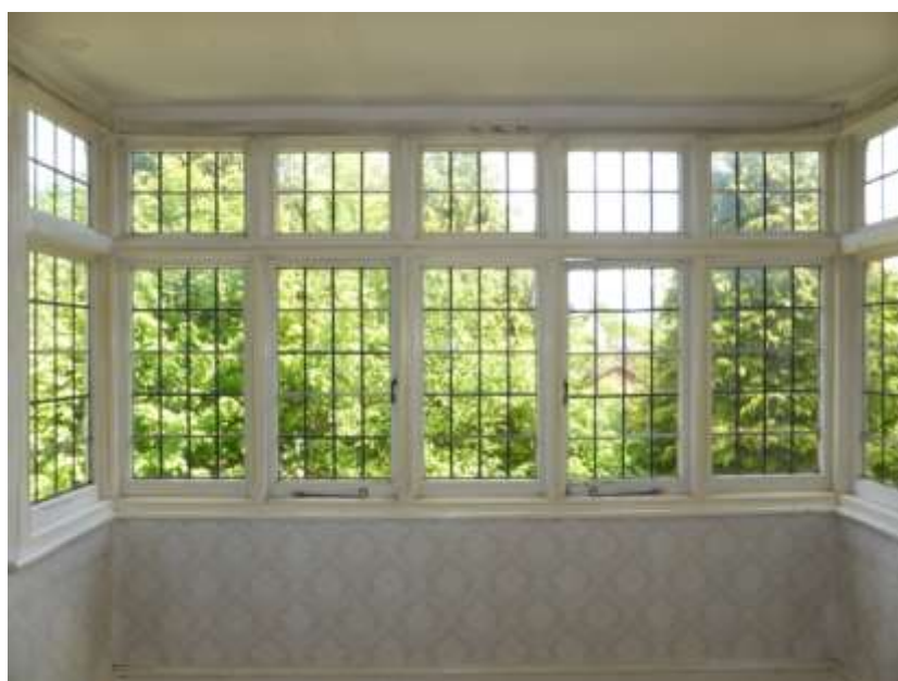
Figure 53: Detail of the early 20 th century leaded lights to the oriel window in F5
