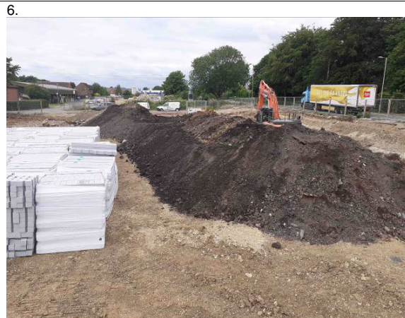
04.06.20 – Soils not demonstrating significant contamination indicators stockpiled to south of excavation area (1/2).
