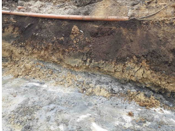
04.06.20 – Soils demonstrating residual indicators of contamination present within northern sidewall of excavation; unable to progress excavation northwards.
