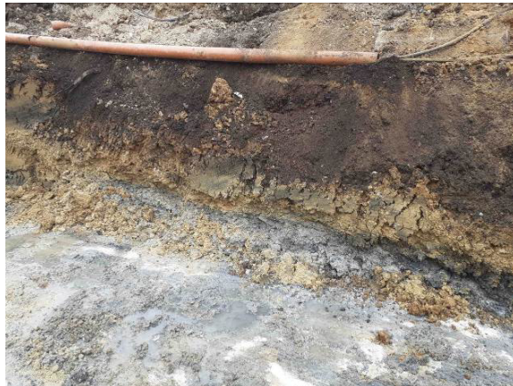
04.06.20 – Soils demonstrating residual indicators of contamination present within northern sidewall of excavation; unable to progress excavation northwards.
