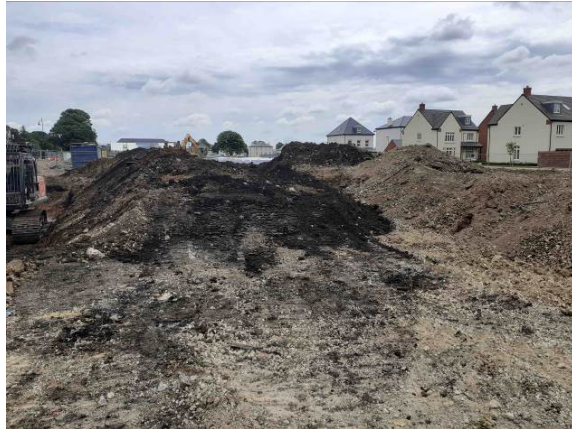
04.06.20 – Soils not demonstrating significant contamination indicators stockpiled to south of excavation area (2/2).
